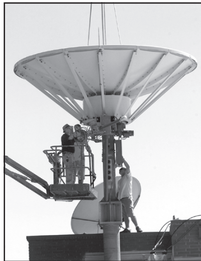
The CCCSAT team works on the uplink equipment at Palomar College
